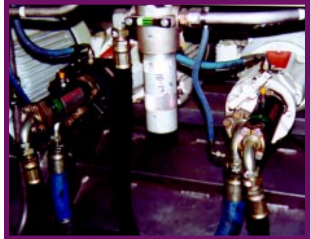
Shown are two suppressors mounted on the front face of two pumps. Before the suppressors were added this was a noisy installation because the steel floor under the pumps radiated the noise.
