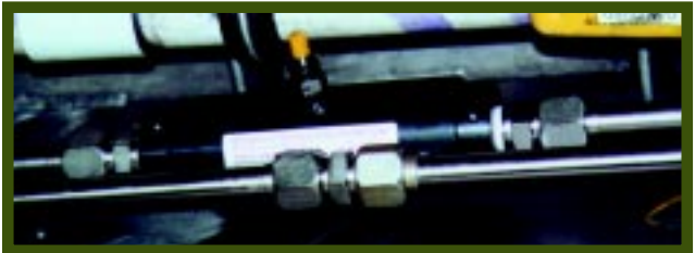
The straight thread suppressor is easily added to a run of tubing. There were two tube joints at this location. One was easily replaced with a suppressor.
