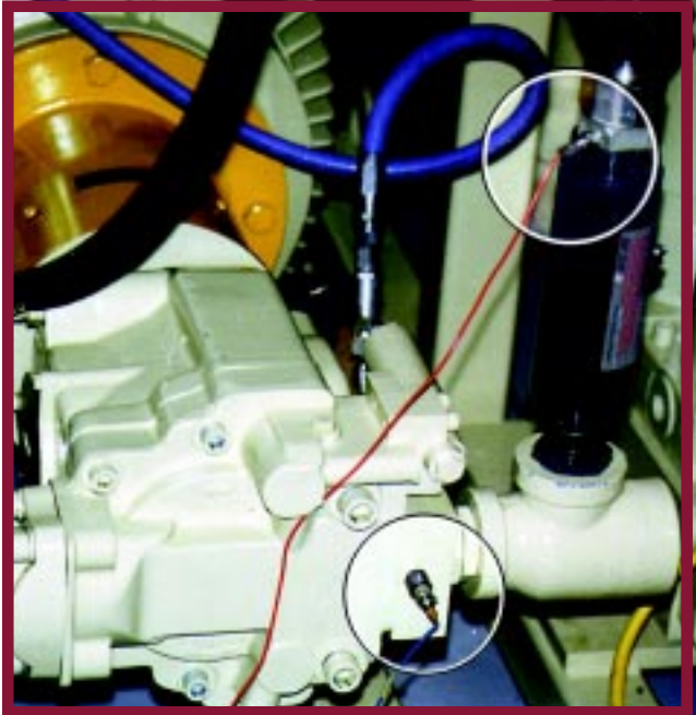
This photo shows the Suppressor mounted at the pump outlet. There are sensors mounted immediately before and after the suppressor leading to the oscilloscope. This is the method used to get the tracings shown below.
