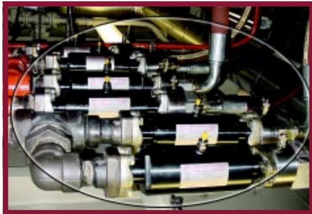
Due to space configuration, these six Suppressors were mounted in the lines leading from the pumps.
